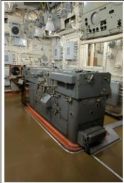
The Fire Control system on HMS Belfast
