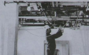
Walsall trunking, cable tray and conduit being installed in a corridor ceiling.
